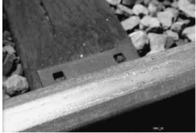
Figure 22. Top of rail 4 weeks after coating, showing film flaking off rail.
